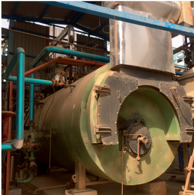
Figure 8. Combined boiler used in the chlor-alkali factory.
